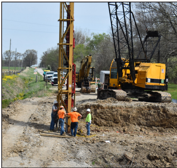
BRIDGE WORK PROGRESS: The NE 301 Road bridge is currently being replaced by members of Haile Excavating (who won the BRO project bid); Haile Excavating is out of California, MO. who can be seen here starting on one of the pilings. The old bridge structures have been removed.
