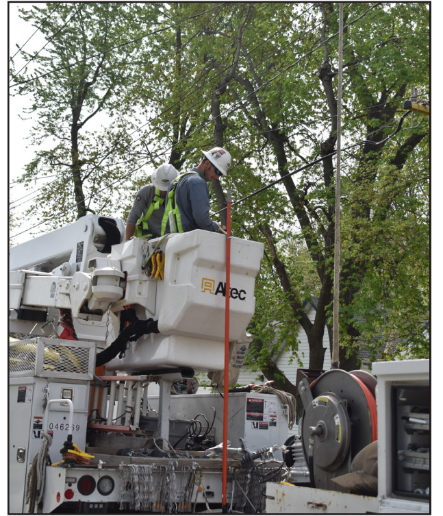
EXPECT DELAYS AND DETOURS: Intren, subcontracting for Evergy, is repairing, replacing lines, and also replacing utility poles along the Green Street roadway. The work is expected to take a few months and also incorporate utility lines and poles along Seventh Street towards Casey's.
