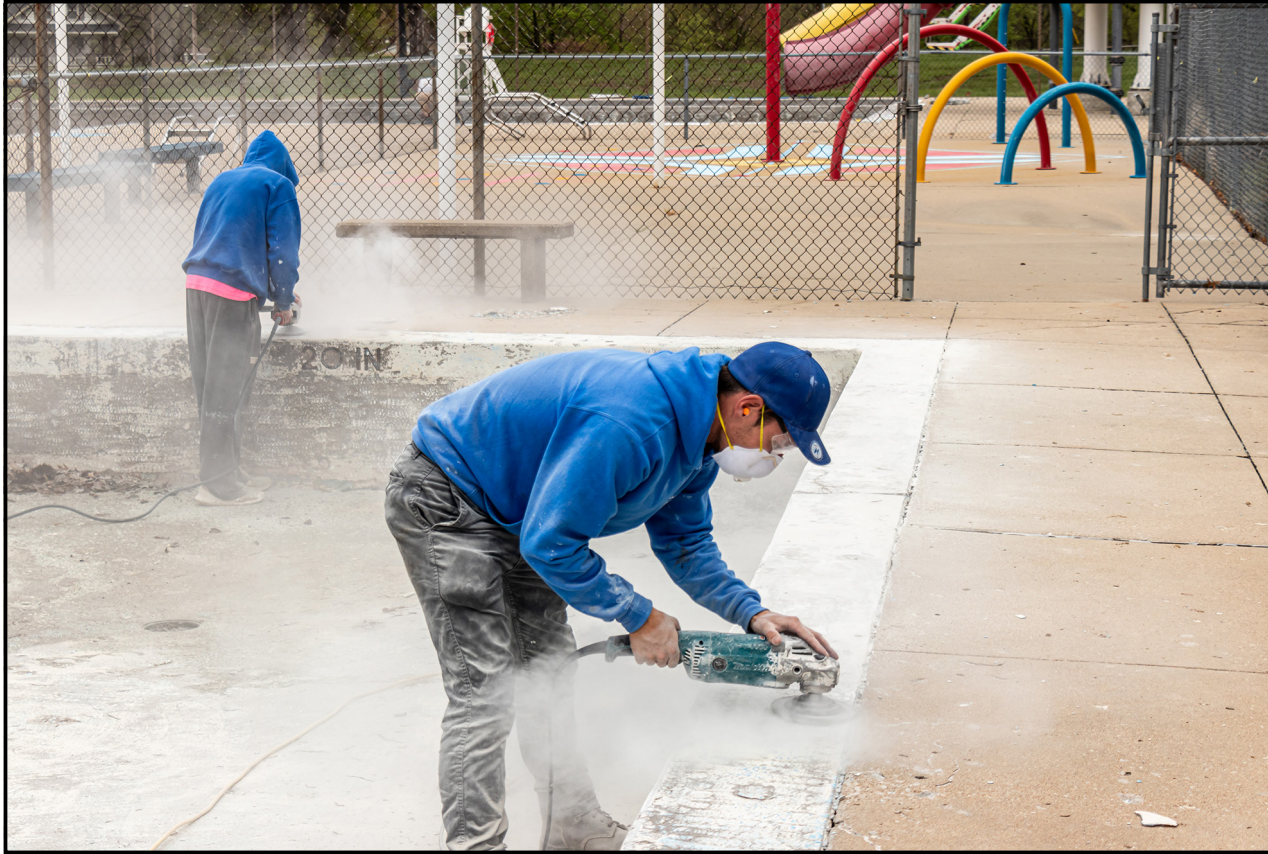
PREPARING FOR SUMMER SWIMMERS, Logan Colman and Caleb Martin worked on re-opening the Clinton pool at Artesian Park on Monday. They are employed by Mid-American Pool Renovation.
