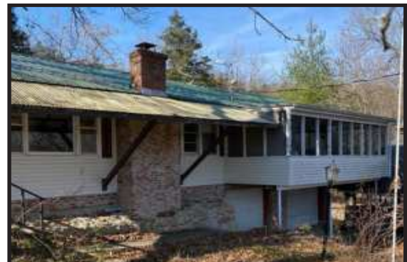
RESORT HOME WITH LOTS OF POTENTIAL! Inside needs finished. Some of the sheet rock is in place with some items for repairs. Newer central air and heat has been installed. Nice 2 car garage. Lake view. On blacktop road. Nice area! Call Julia today and take a look! $162,000 MLS#93479
