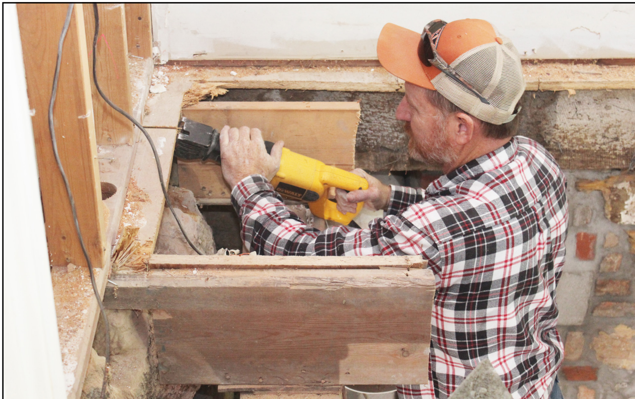
BRINGING THE STORIED DORMAN HOUSE BACK TO LIFE, Pete Owenby worked on the sub-floor joists in the music room where a new concrete floor was poured.
