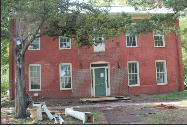
THE BRICKS WALLS of the Dorman House are now stabilized. Phase Three calls for removing the paint on the bricks and covering them with a breathable finish.
