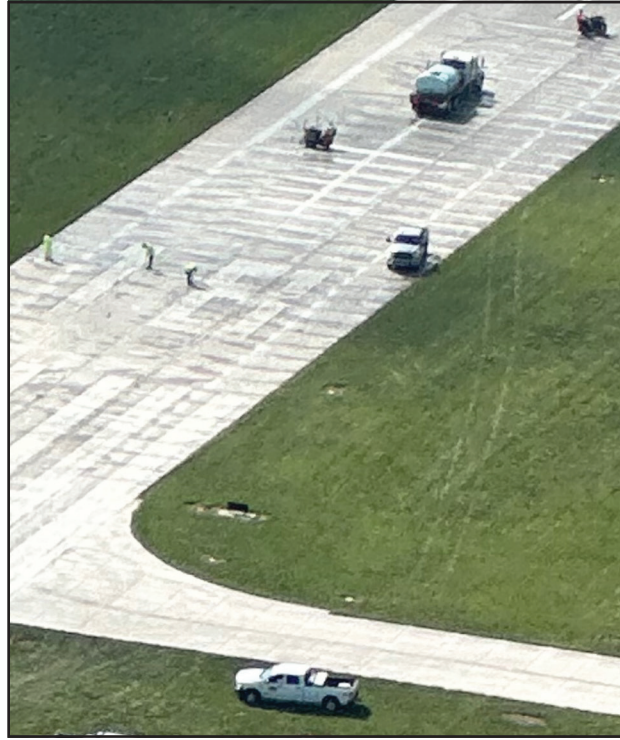
AN AERIAL VIEW of the grind-and-seal work being done on the expansion joints of Runway 18/36, the main runway at Clinton Regional Airport, which will make for smoother landings.
