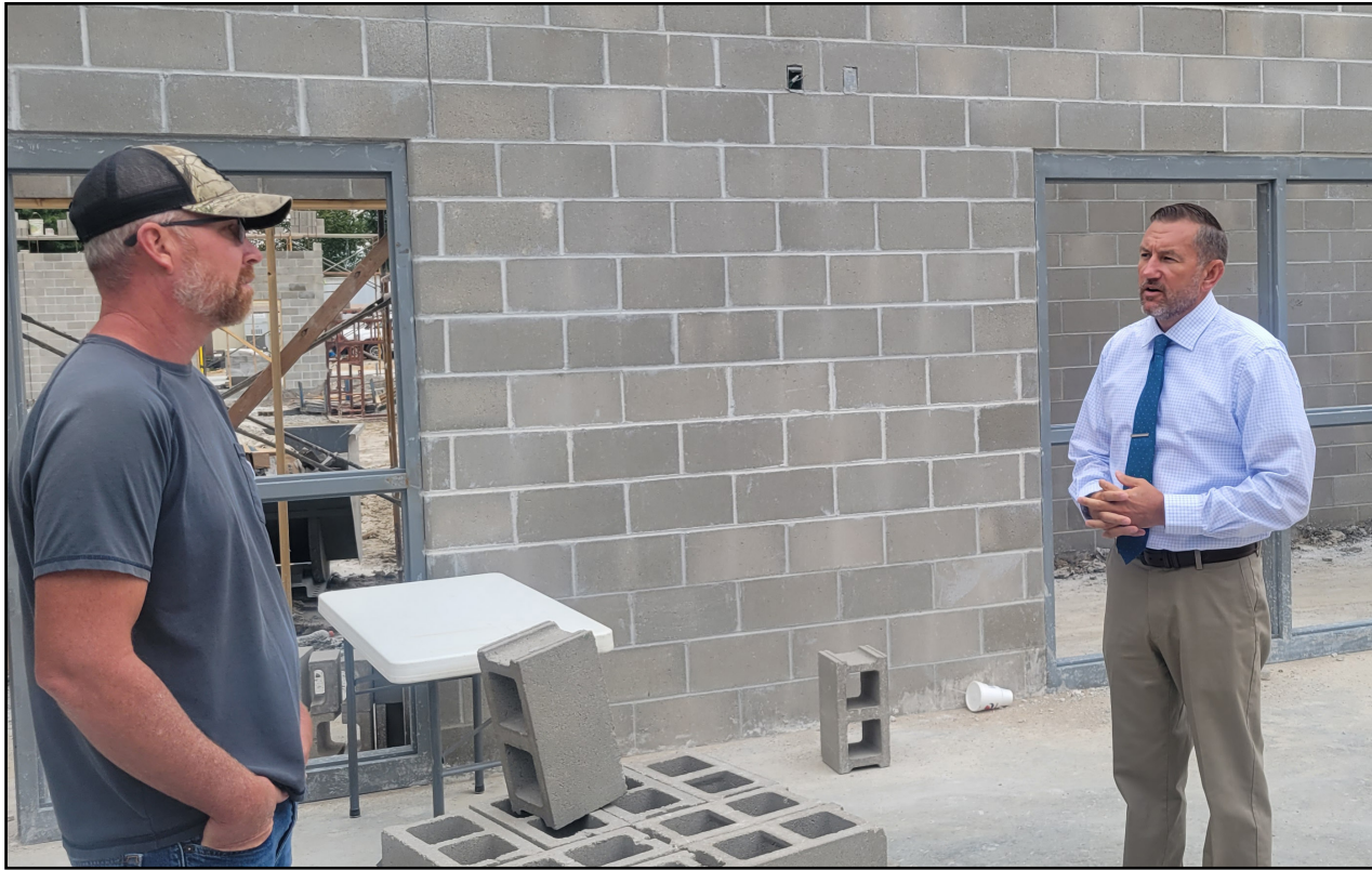
SET TO DEBUT IN 2024 , a massive new addition to Lincoln's R-II campus continues. Superintendent Kevin Smith and School Board Member Jason Smallwood did a progress check on Tuesday morning.
