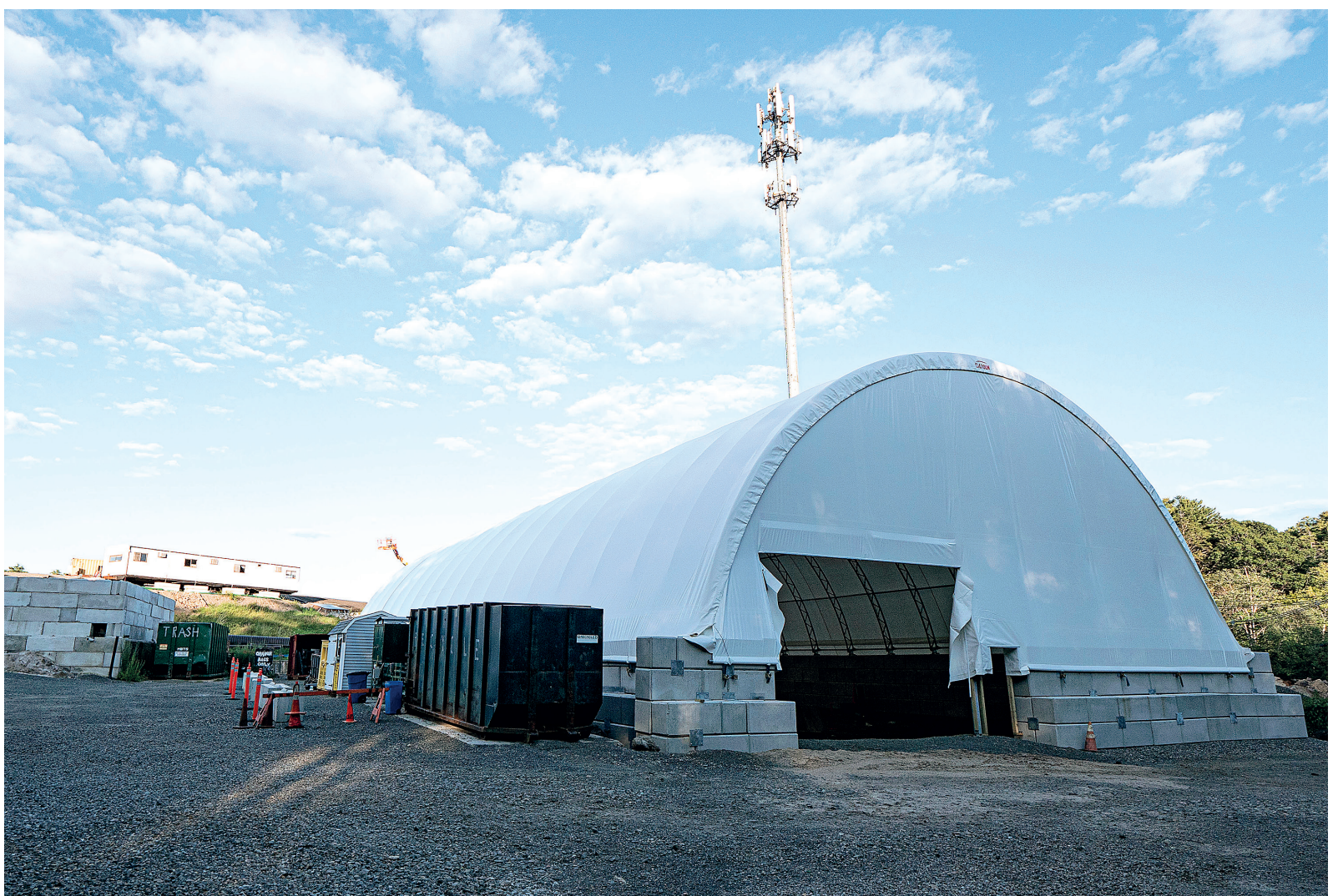
Wow! Black Earth Composting's new home on Pine Street in Manchester is taking shape quickly, with a domed structure that will process more than 28 tons (that's more than 56,000 lbs) of food waste per week from across Northeast Massachusetts in this state-of-the-art facility, expected to be up and running in Spring 2024.
