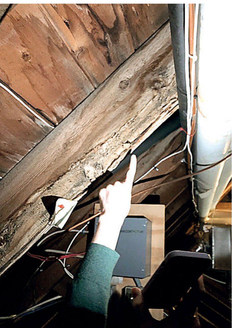
Photo illustrates water damage to Manchester Public Library rafters that was exacerbated after two separate severe rain storms.
