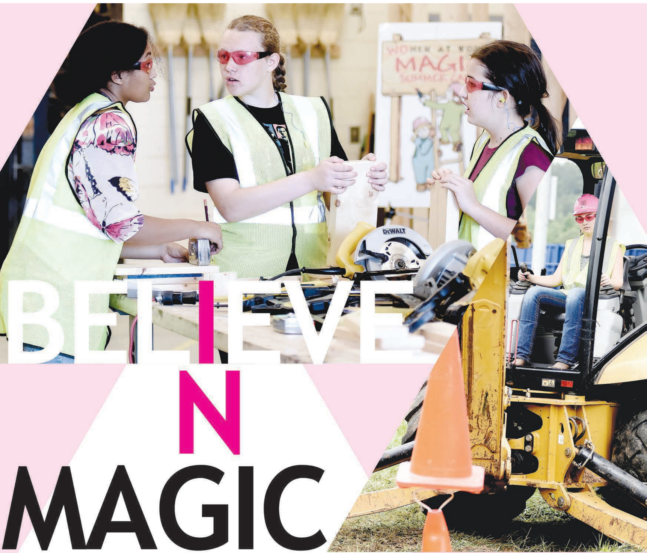
PHOTOS BY RANDY PARKER, DESIGN BY ERIC DEMPSEY Top, from left, Katherine Miller, Sarah Brownlee and Jazmyn Hughes share construction ideas at Magic Camp at Cass High School. Above, Julia Stein learns to operate the bucket of a backhoe. Bottom left, Gabrielle Woodside uses a router to smooth wood. Below, Stein operates a blow torch.
