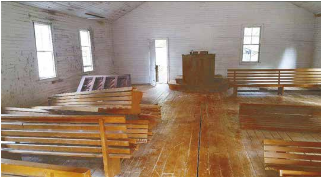
Numerous pews found damaged in the church.
