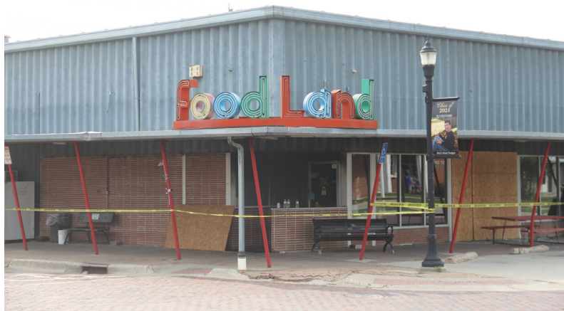
A fire at Food Land in Woodbine on Aug. 19 has forced the temporary closure of the local grocery store. As shown in the photo, the building is not a complete loss.
