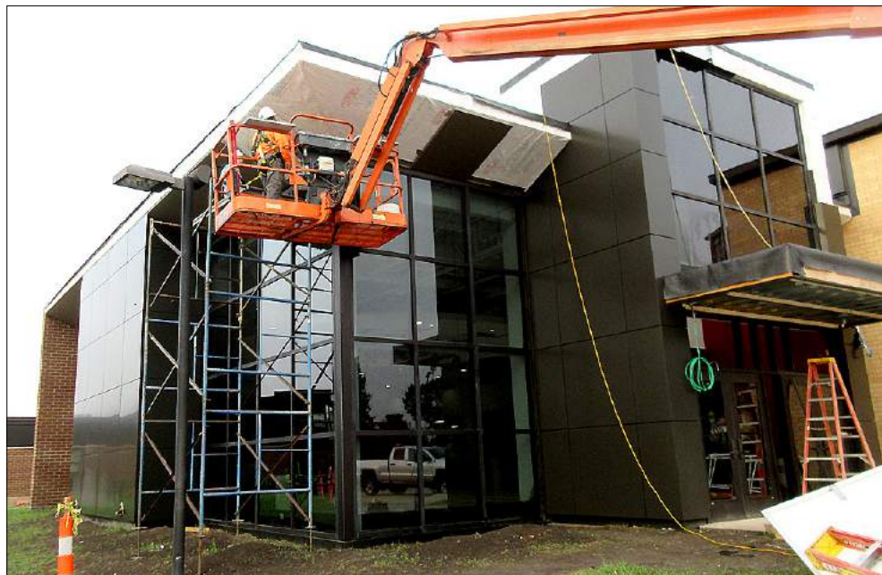
Construction crews affix panels to the front of the auditorium. NSP photos by Bill Tubbs
