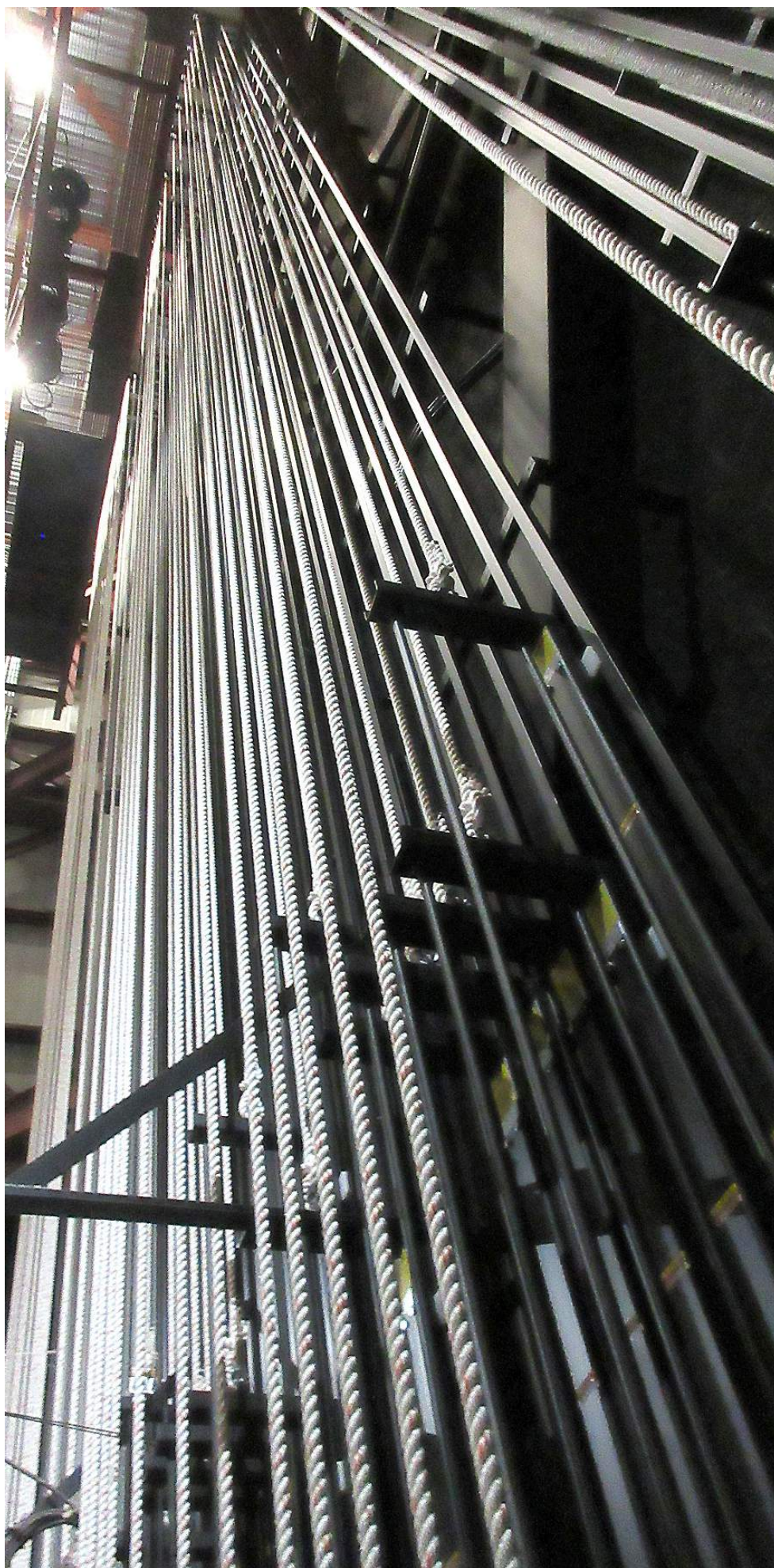
Lines have been added to the rigging for greater function and safety.
