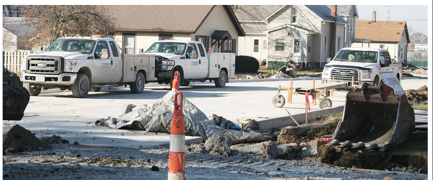
The reconstruction of West Otis Street between Main Street and Rowe Lane in Walcott, shown Nov. 15, is nearing completion. The project, which involved the concrete paving of the street, also included sanitary sewer replacement, a new storm sewer, water main replacement and parking areas for Wescott Park and the Walcott splash pad. Funds from the city's road use tax and local option sales tax are paying for the reconstruction project. The splash pad, to be located on city-owned green space just east of the community's batting cage and tennis courts on West Otis, is scheduled to open in next summer.
