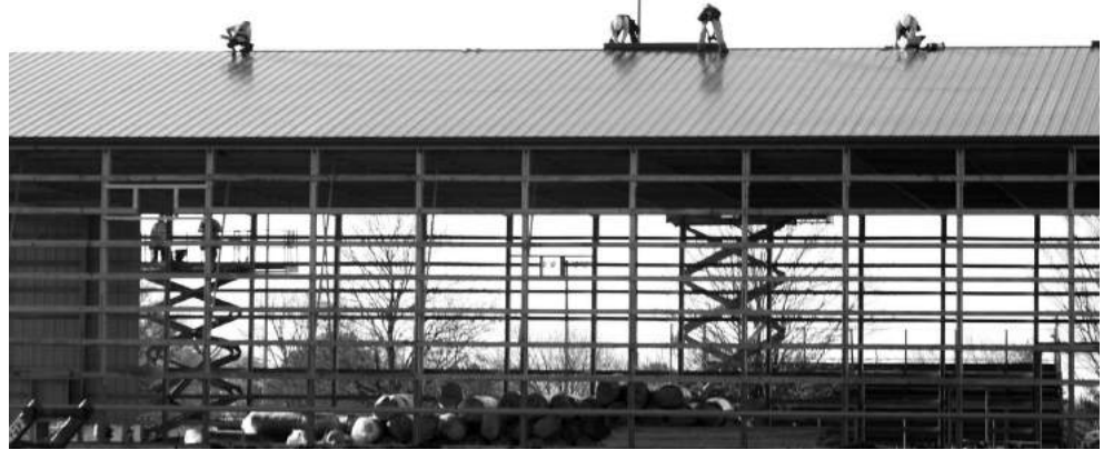
Contractors in 2019 build the indoor practice facility to replace the Silver Bullet.
