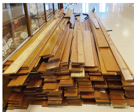
The original wooden bleachers were removed from the Durant High School gymnasium, making way for new, blue resin plastic bleachers installed in the summer. Materials for the new bleachers are shown (left), encompassing the gym floor June 4. The wood from the old bleachers (above) was auctioned off.
