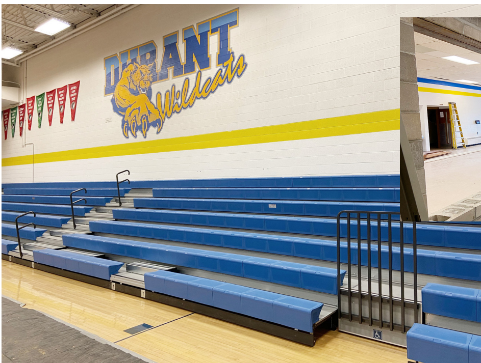
The new blue Durant bleachers were installed in July, replacing the original wooden bleachers in use since the 1970s. Above, the south-end storage room was converted into a new concession stand. Shown are the two openings and storage area in the new concession stand
