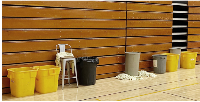
The Durant School District approved a bid in March to repair all remaining district roofs that were leaking, including the high school gymnasium, which began seeing significant leaking in the spring due to heavy snow melting. Buckets are shown in the gym, used to collect water.
