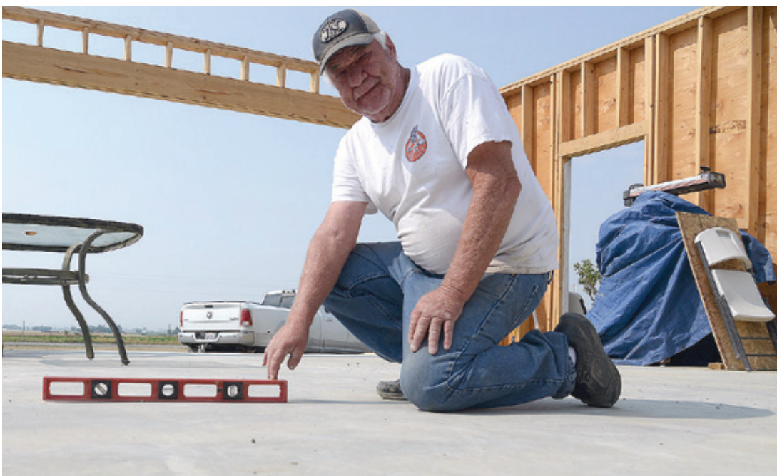
Stan LaBlue uses a level to show the slope of the concrete in the unfinished garage he paid Wiggins Construction to build. He and his wife, Debbie, paid the company over $90,000 to set up their house and build a garage and patio. Very little of the work was completed and what work was done, the LaBlues claim, was substandard. Tribune photos by Kevin Killough
