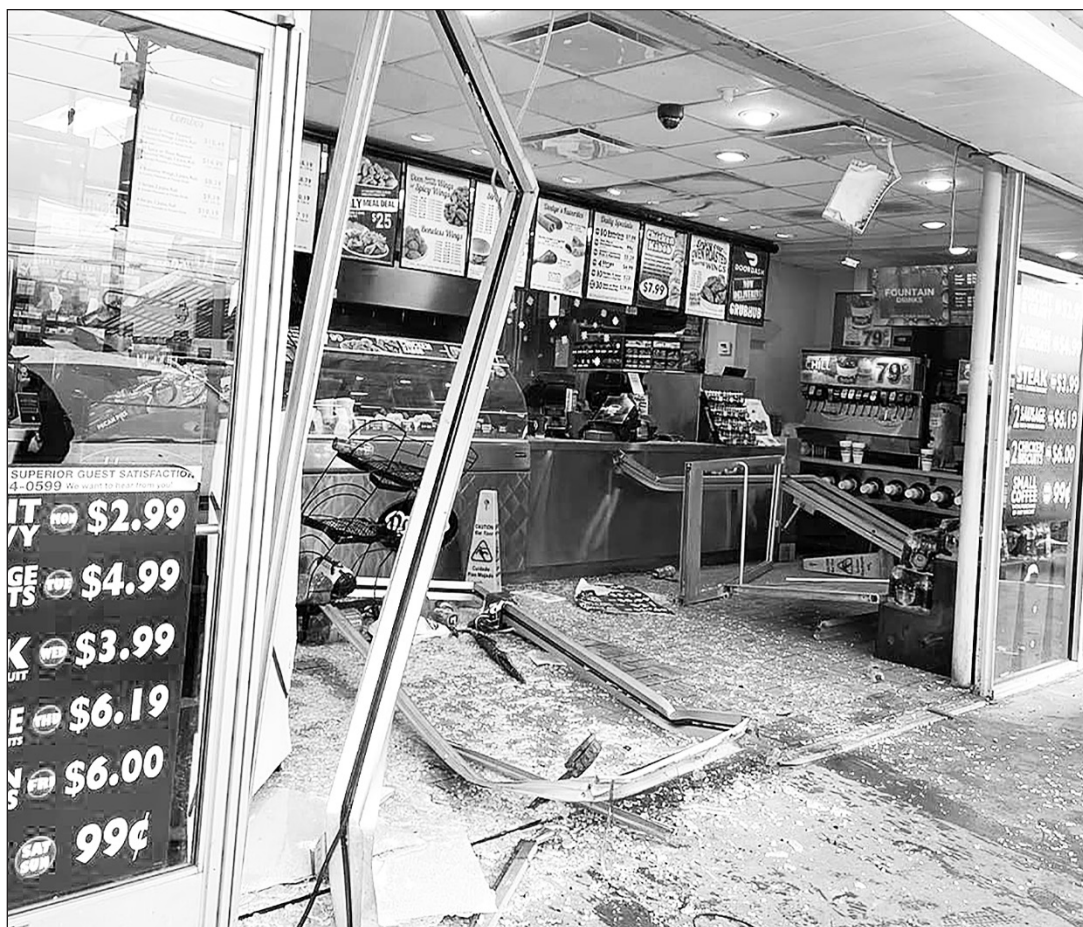
A Savannah Police Department photo on social media shows damage at Dodge's Store caused when a vehicle crashed through the building on Saturday, Jan. 7.
