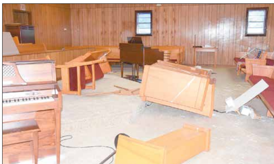
VANDALIZED - This is the pulpit area of Obion River Association Headquarters in McKenzie that was vandalized recently. Furniture was overturned, paint and cleaning supply contents were poured all about on the carpet and on a number of seats as well as other areas. Photos by Shirley Nanney
