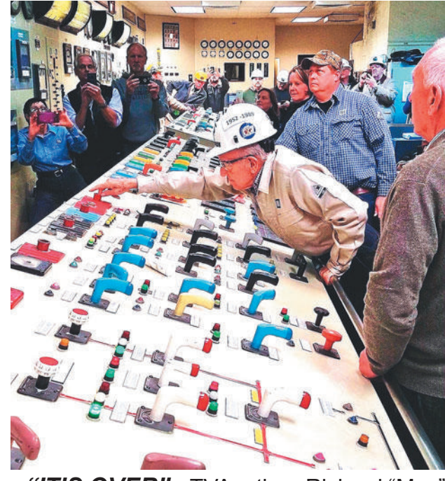
"IT'S OVER" - TVA retiree Richard "Mac" Flowers, 91, was joined by other Johnsonville Fossil Plant employees as he opened the breaker to separate the plant's last operating unit from the grid on Sunday, Dec. 31, 2017, at 7:14 p.m. CST.
