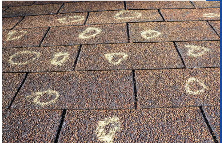
Insurance adjuster marked roof with hail damage
