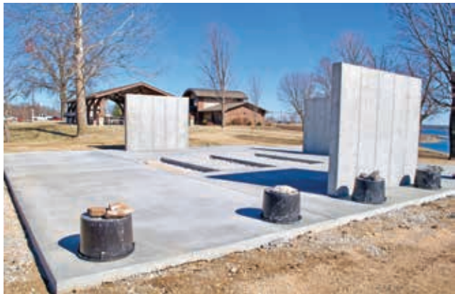
Concrete foundation has been poured for the Stockton Veterans' Memorial Park, which is set for a May 21, 2022, grand opening. STAFF PHOTO/KATHRYN SKOPEC
